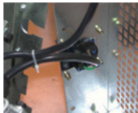
[5] Affected fan - rear of electrical socket & conductors
