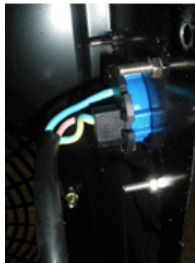
[6] Affected fan - rear of electrical socket &
