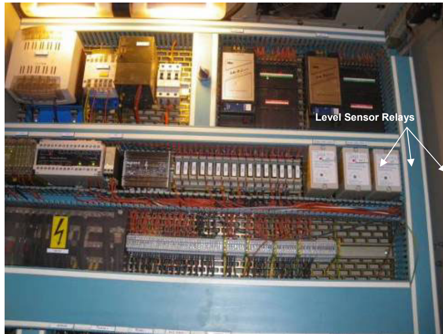
Level Sensor Relays in Electrical Control Panel
