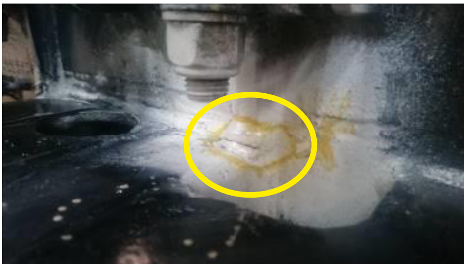
▲ Strengthening gusset cracking below seat
