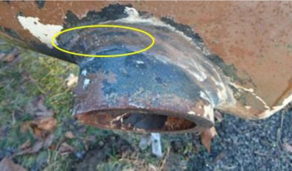
Lower support leg bore circ welds cracking (visual & mpi)
