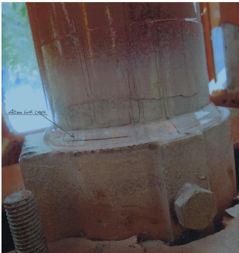
40mm long crack
